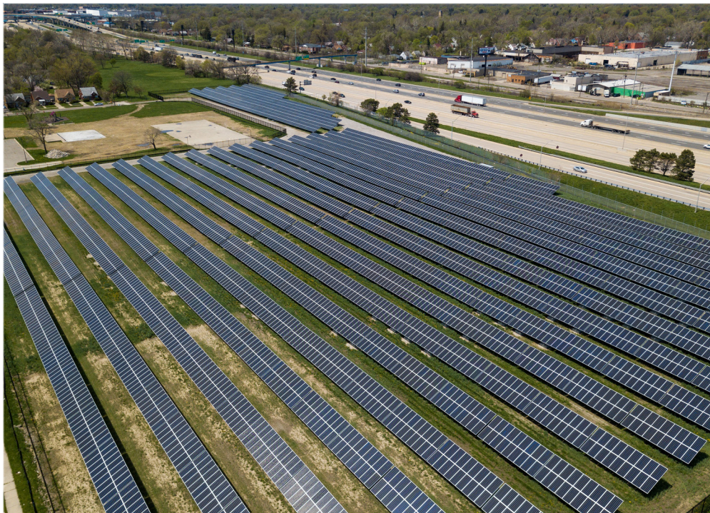
Solar field in Detroit | Courtesy of DTE Energy
